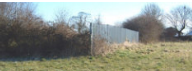
Security railings, Adel St John's School boundary with the Bedquilts Playing Fields
